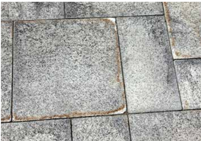
Paver damage and rust from metal plow blade
