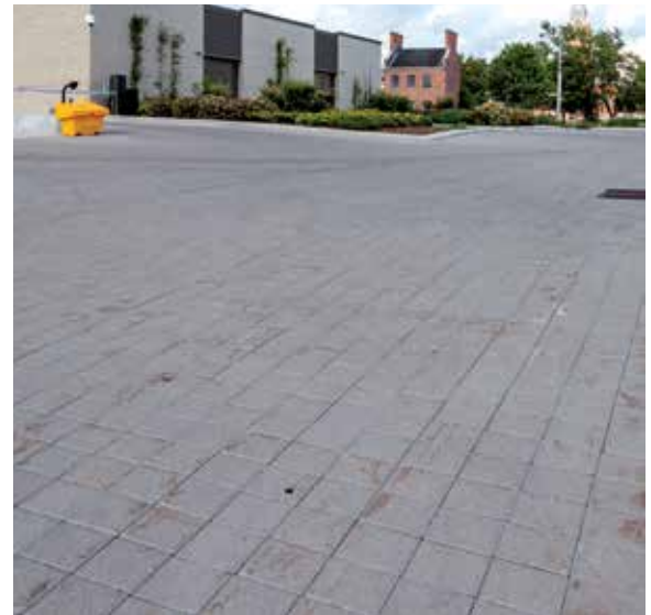
Rust marks on pavers from metal blade plow
